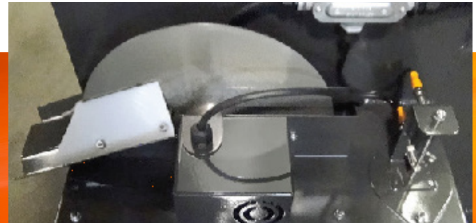
Oil Skimmer and Tank Low Level Switch
